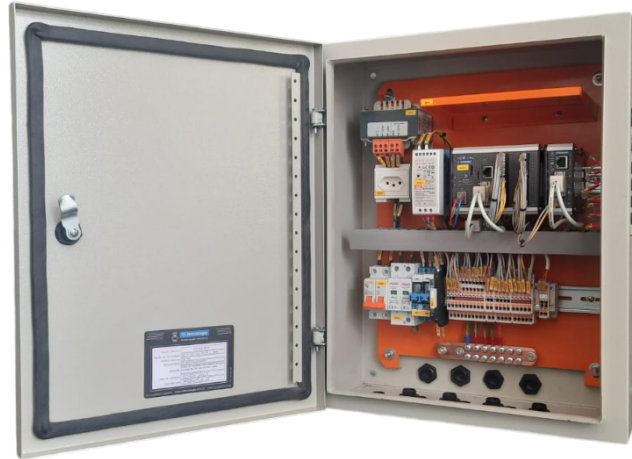
Figura 1 - Painel ACOS225 BCS STD com Gateway Modbus, vista frontal
